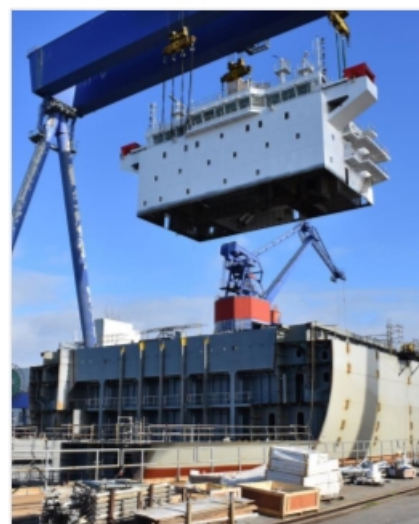
Installation of the house on the Kaimana Hila at the Philly Shipyard, August 2018.
