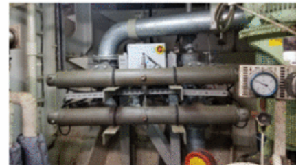
Ballast Water Treatment System
