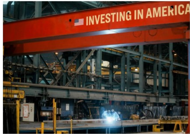
Cutting of steel at the Philly Shipyard in Pennsylvania initiates the construction of our three new “Aloha Class” vessels
